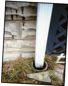
Example of inflow: A downspout connected directly to the sanitary sewer system.
